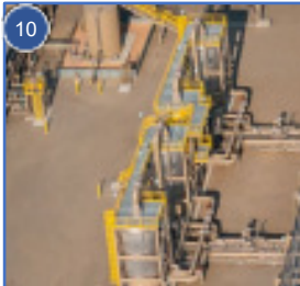
10 H2S TREATING Removes Hydrogen Sulfide from the inlet gas stream
