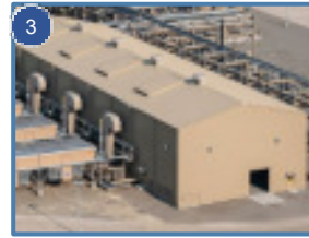
3 RESIDUE GAS COMPRESSORS HP compressors per processing train raise the processed residue gas pressure up to residue gas delivery pressure
