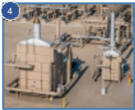
4 HOT OIL HEATERS Natural Gas Fired process heaters used to increase the temperature of heat transfer fluid (hot oil).
