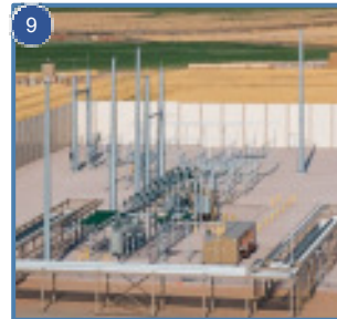
9 ELECTRIC SUBSTATION Power from local utility is stepped down through transformer for use in the plant.
