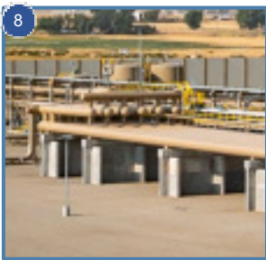
8 HIGH PRESSURE SLUG CATCHER Receives high pressure gas and slugs of NGL liquid from the high-pressure gas gathering system.
