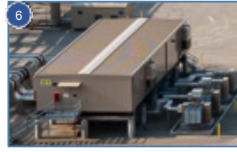
6 POWER DISTRIBUTION CENTER Distributes electrical power to the various electric powered equipment in the plant.
